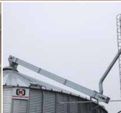
KCA chain conveyor for inclined conveying along silo roof
